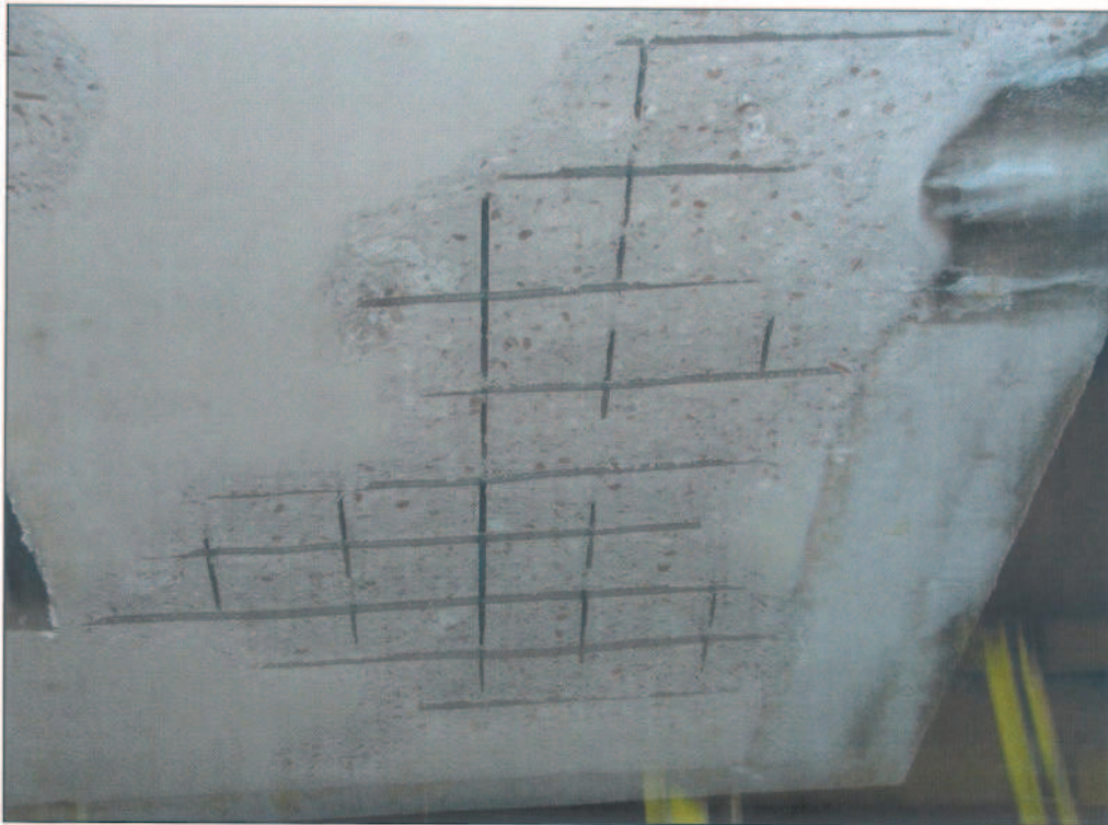
ES of supporting structure – reinforced concrete panel after the finished test of fire resistance
