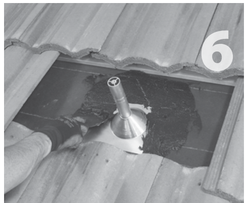
Apply 1/8" thick layer of roofing cement around the top and sides of the subflashing with at least 1" extending past the sides of the flashing onto the felt. Layer should be about the thickness of a nickel.
