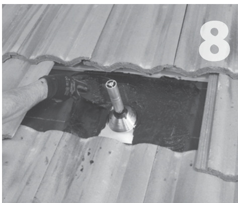
After first layer of cement is dry apply second layer of subflashing over reinforcing fabric to finish waterproofing of subflashing.
